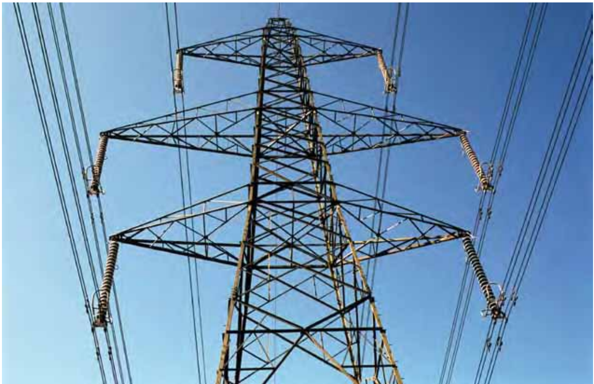
The UK will need a bigger, smarter electricity grid for the future
